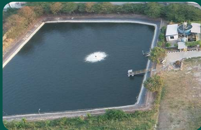
Fasilitas Clean Water Treatment
